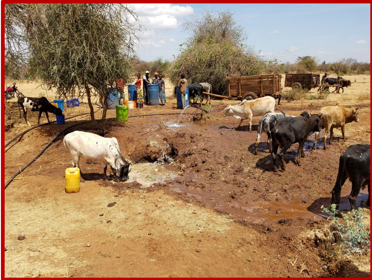
Figure 7: Cows rush to the freshly tapped water supply in Ghalunyangu village following water pump installation in November 2018. Image credit: Scott Shearer.
