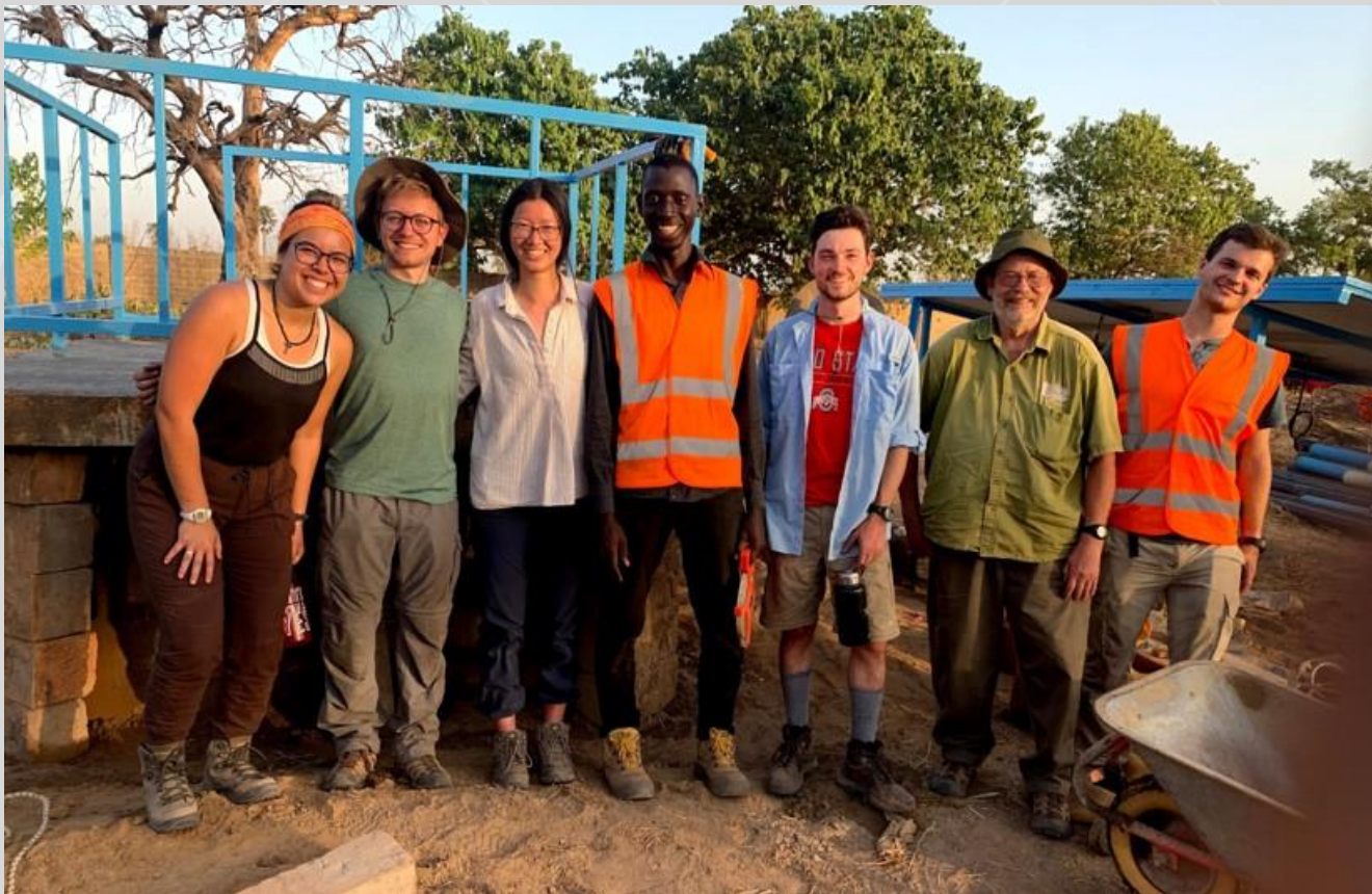
Engineering Without Borders members from Ohio State visited The Gambia for project implementation. They drilled a borehole, capped the well, created a water tank stand, and installed solar panels for the pump
